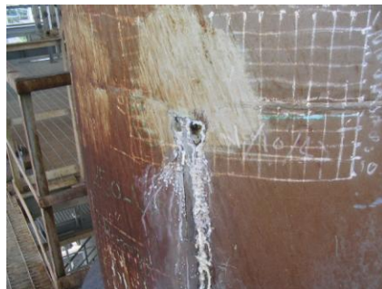
Figure 1: Incoloy 800 pipe leakage by corrosion attack.
