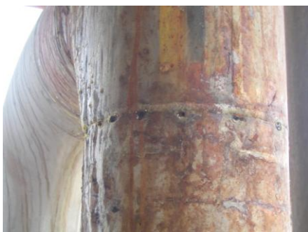
Figure 2: Corroded holes at HAZ of the Incoloy 800 pipe after 9 months of service.
